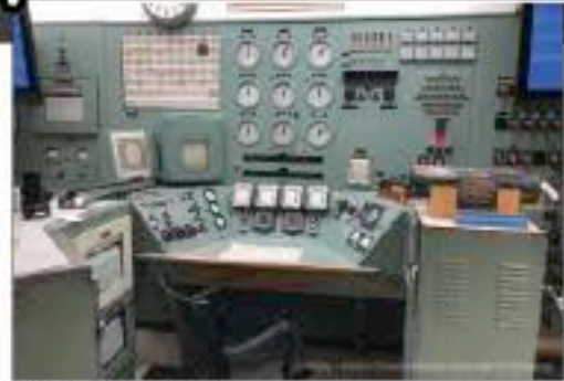
B Reactor control station.
