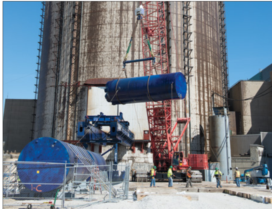
Lessons learned resulted in steam generators being removed twice as quickly from the Unit 2 reactor (3 months) as Unit 1 (6 months)
