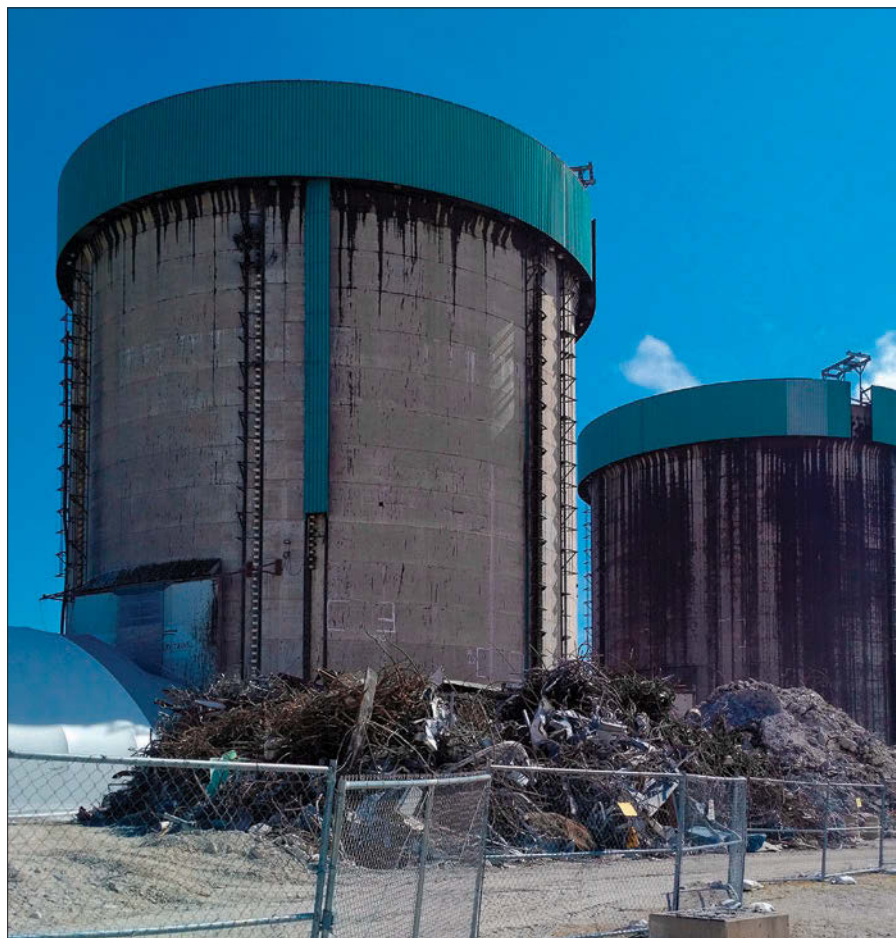
Zion: Lessons learned from segmenting, packaging, and transporting waste are being transferred to other D&D projects.
